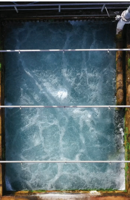
Water purification tank.
